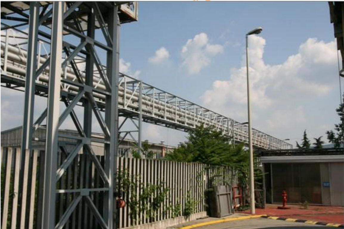
Img 2. Steam Pipeline
