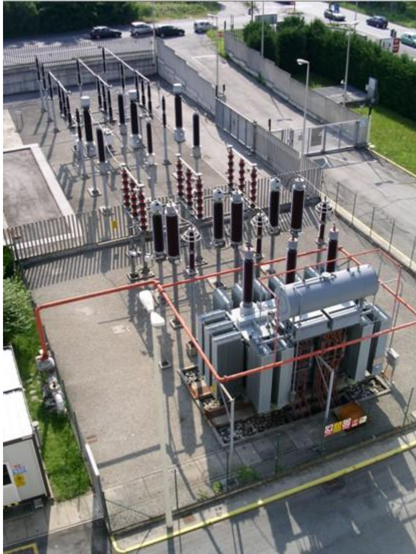
Img 7. External view of the transformers
