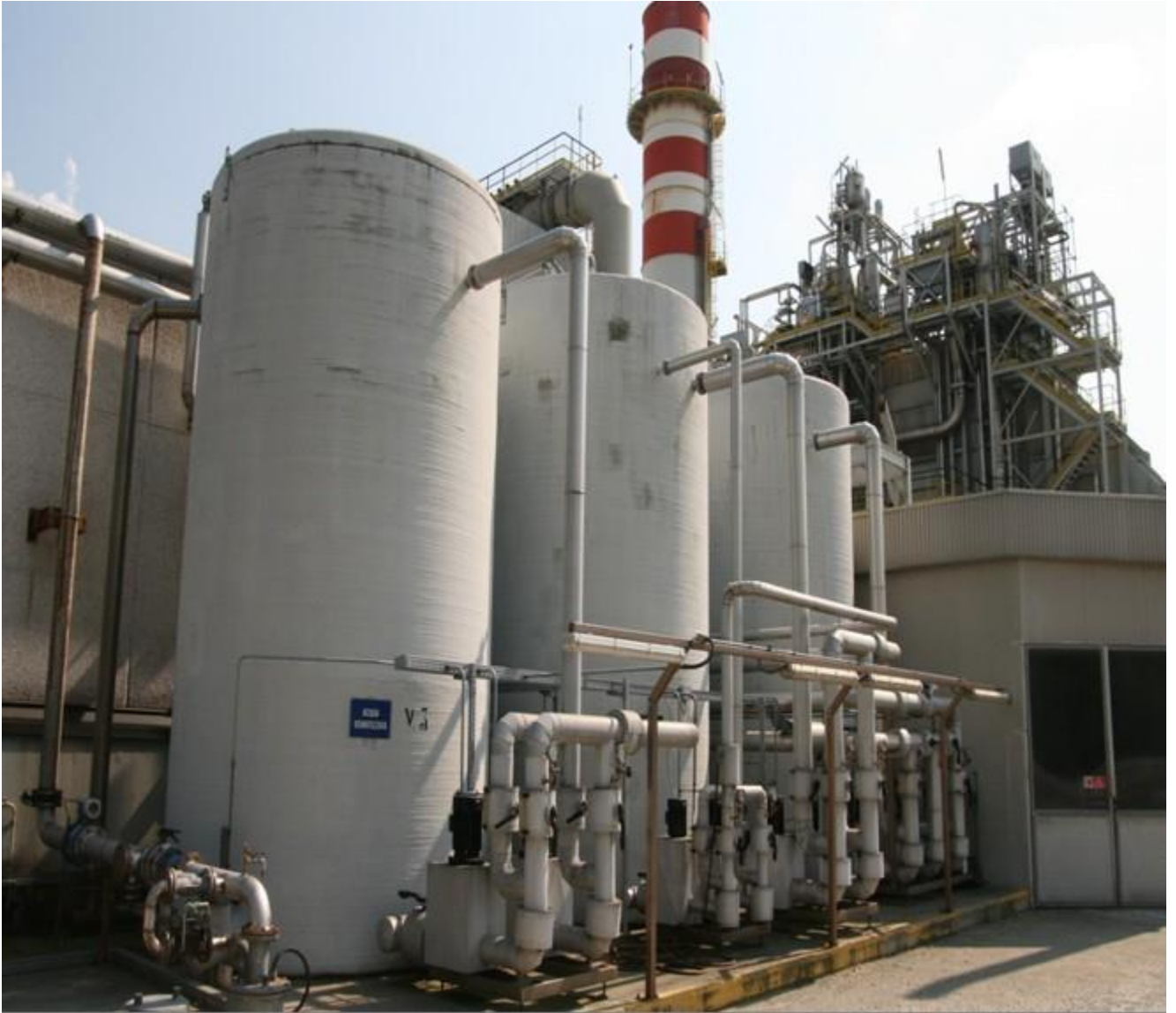
Img 6. Demi-water tanks
