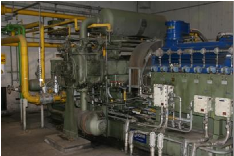
Img 1. Compressors room
