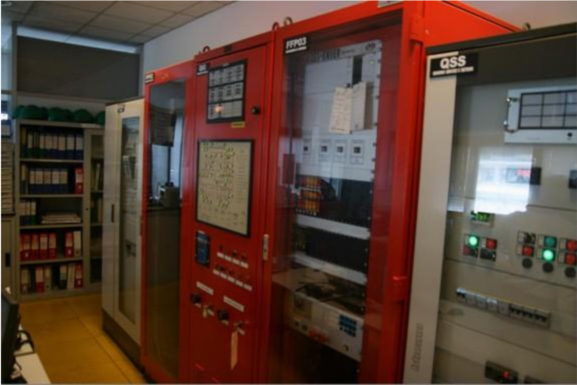
Img 10. Control room
