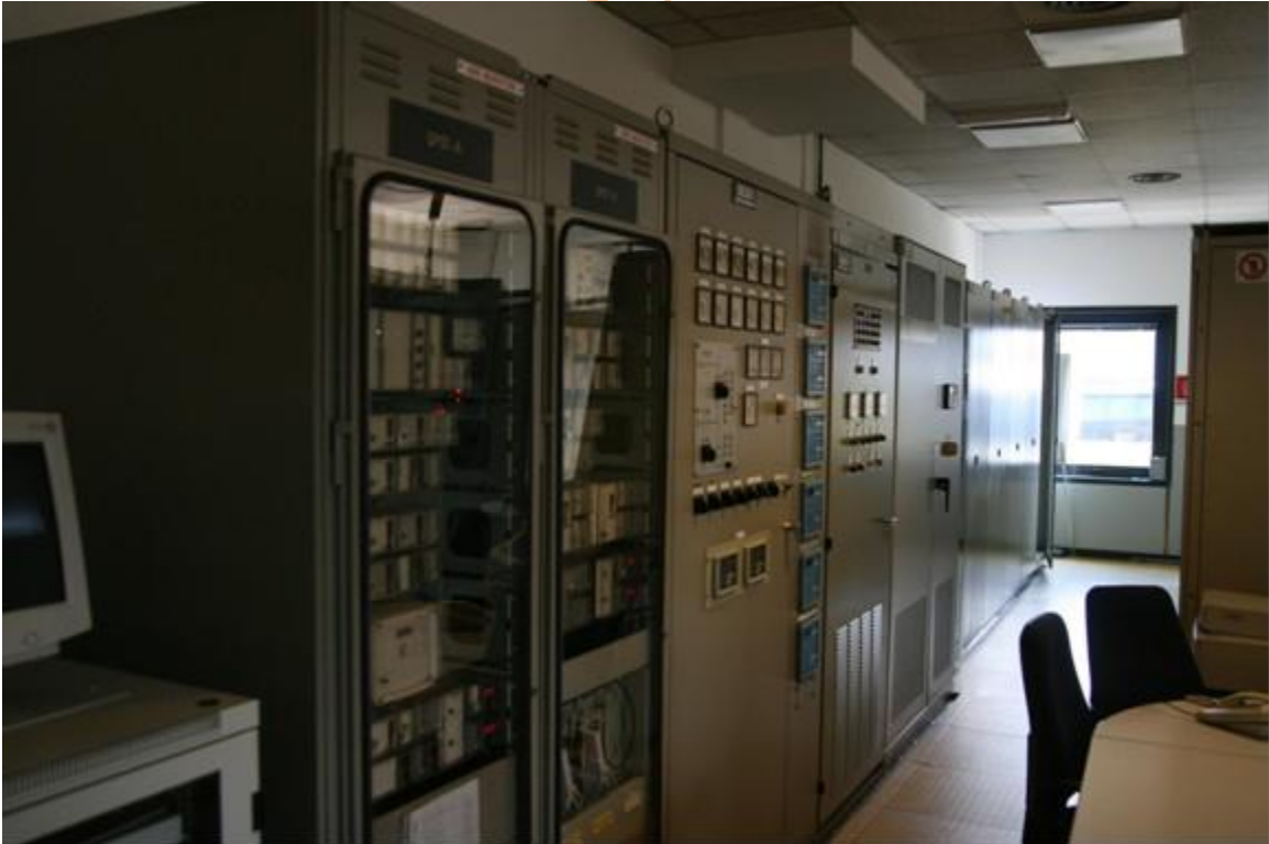
Img 11. Control room
