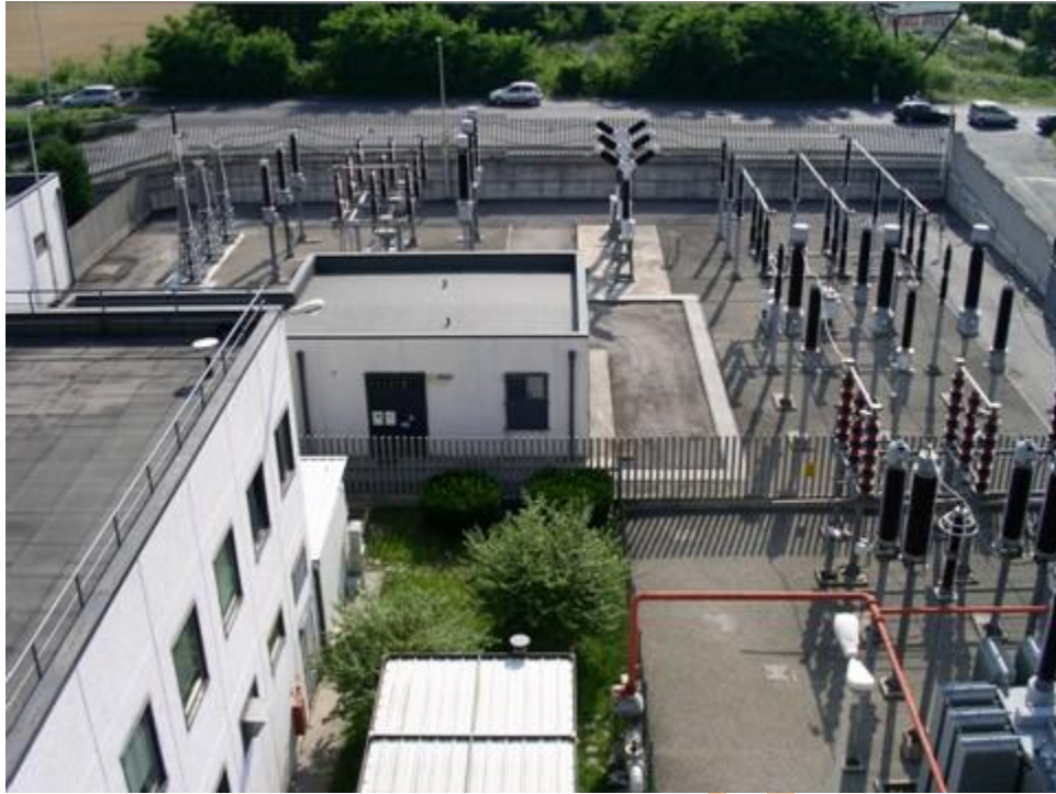
Img 8. External view of the transformers
